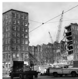
Left: Stetson factory being demolished in 1979. (Michael J.J. Maicher. Courtesy of the Special Collections Research Center. Temple University Libraries. Philadelphia, PA)
